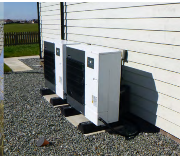
↓ Newly installed heat pumps
